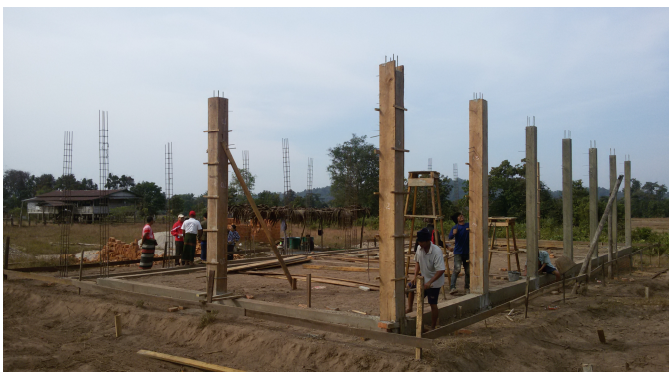
Primary school construction in NgaYitChaungPyar village, Hlaing Bwe township, Kayin State. It was completed in April 2015.
