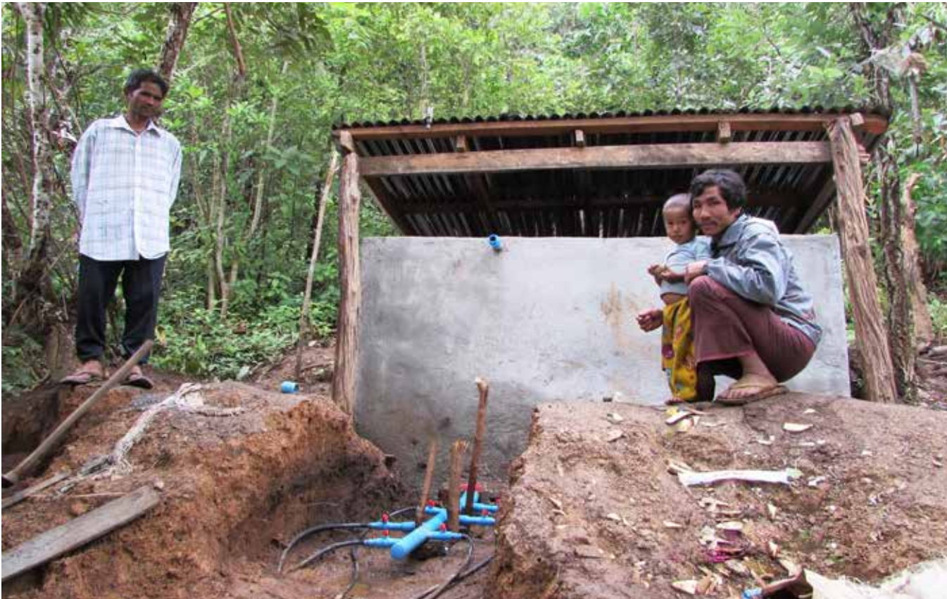
U Shwi Har, VDC's treasurer standing next to the new water supply system at Shane village, Mindat Township, Chin State.
