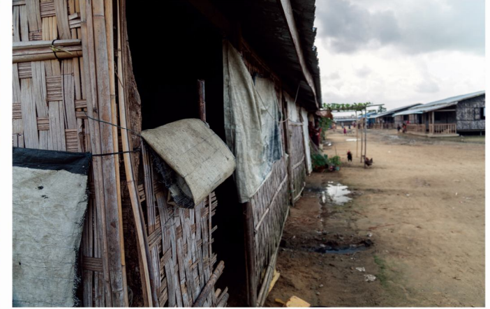
For nearly two years, Ohn Taw Gyi South, Sittwe, Rakhine State has been a temporary home to hundreds of families. People's lives are cramped and without privacy, living in these long and dilapidated bamboo houses.
